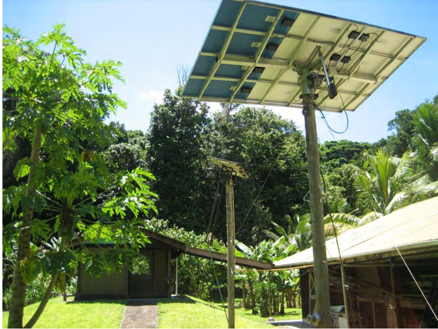
Generator room, solar panels and back of workshop
